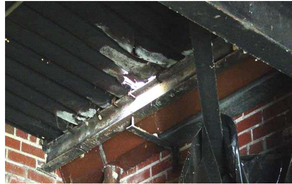
Figure 2.67 Hole in roof of pumping station. (IL)
