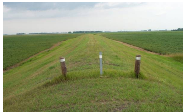
Figure 2.5 MINIMALLY ACCEPTABLE . Field encroaches on levee easement. The landowner has tilled the soil right to toe of the levee, and was requested to stay back at least 10 feet. (ND)
